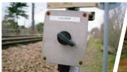
Example of a TOWS switch
