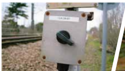
Example of a TOWS switch
