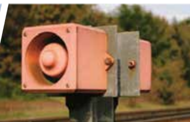
Example of a TOWS warning siren
