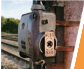
A signal post replacement switch
